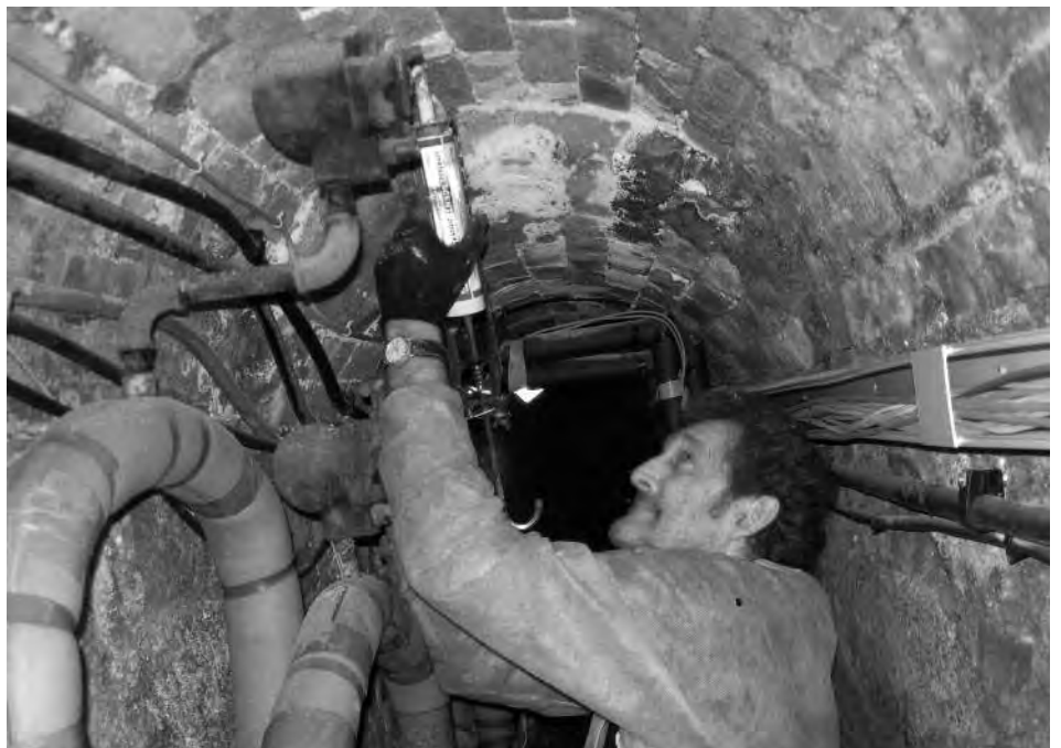
Mick Stone from the Trust's Direct Labour Team seals all breaches from the tunnels into the mansion itself to create a horizontal fire-resistant compartment. © National Trust/Paul Holden
