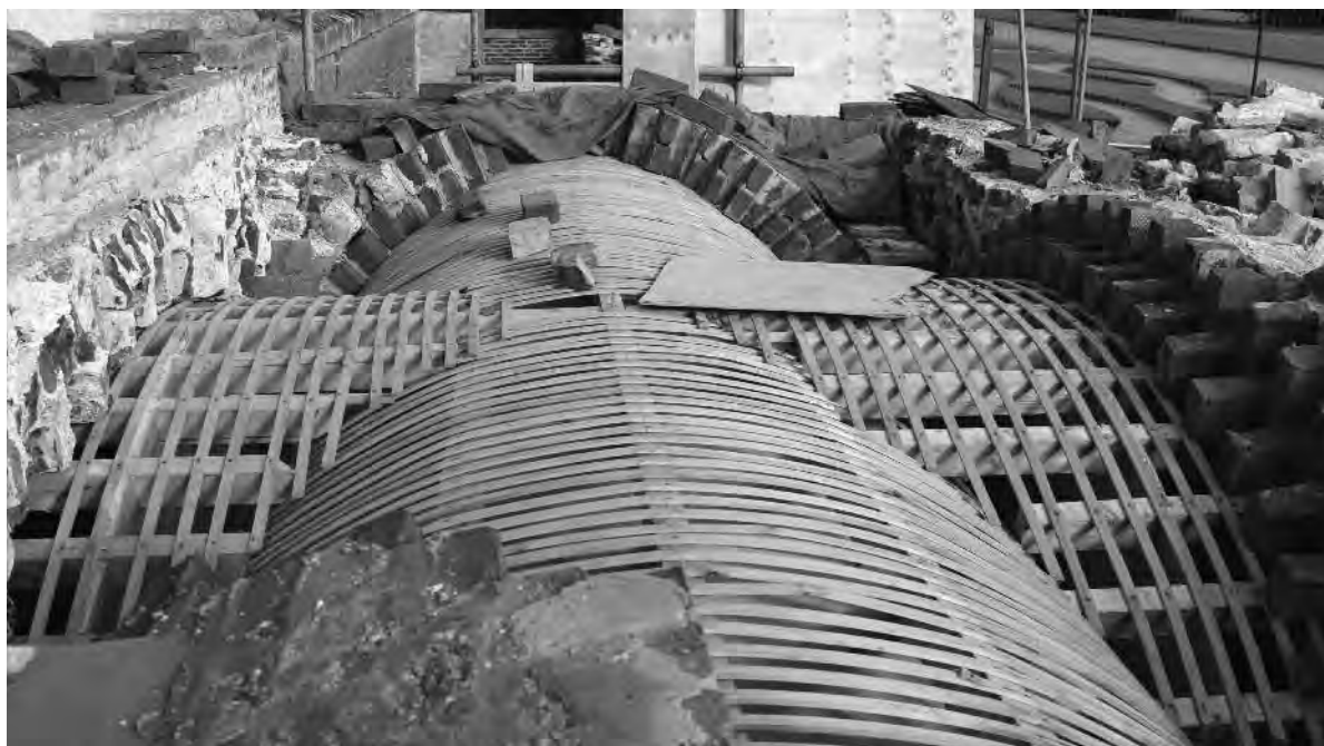
Installation art: the quite beautiful timber former constructed to enable the brick arches of the bridge to be rebuilt, after which the former was dismantled. © National Trust/John Moorey
