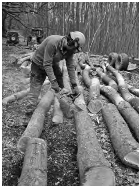
David Elliott, Head Ranger, copping wood for the new building. © National Trust/Matt Bramich
