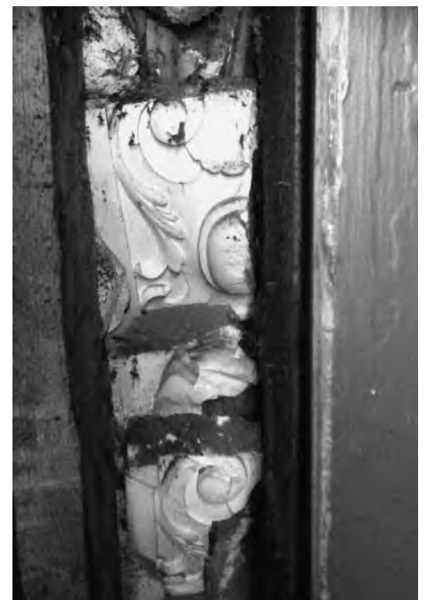
Where compartments were newly formed or upgraded, the door architraves had to be removed to install intumescent seals and foams to prevent any potential fire spreading through the door frames. This caused many challenges, not least as shown here on the Livery Room door case which had been packed full of plasterwork fragments by the Victorians, perhaps to achieve the same ends as modern-day interventions. © National Trust/Paul Holden
