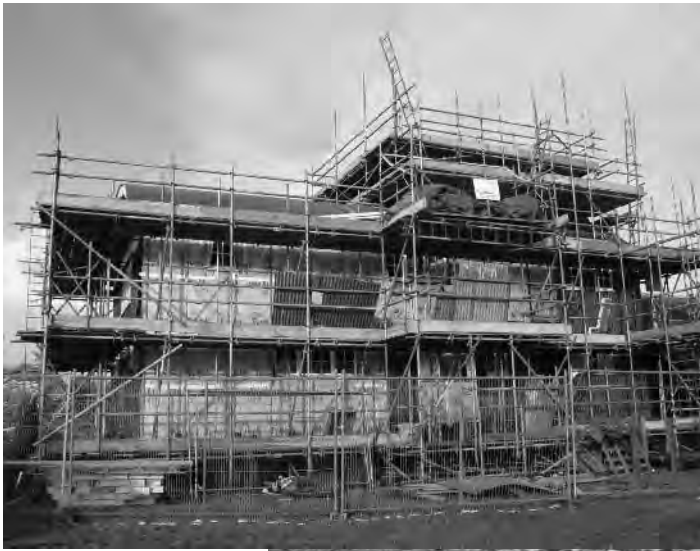
Above: The scaffolding was extensive and robust but the contractors were often unable to work on it because of bad weather. © National Trust/Graham Lubbock
