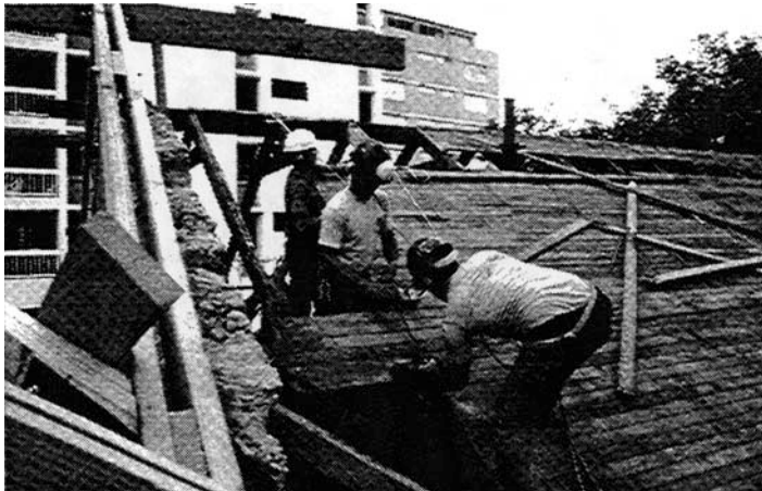
Cutting wood boards before dismantling original roof truss during Colegio de Arquitectos Headquarters restoration in Santurce, PR (19931).
