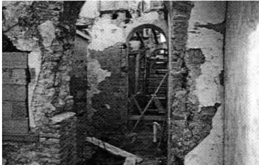
Deterioration caused by the use of incompatible construction materials such as modern concrete block inserted into rubble-masonry fabric.
