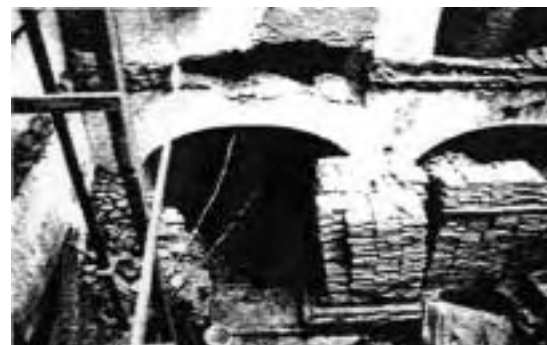
Storage of reusable historic brick conserved from dismantling and selective demolition phase of Casa Ramón Power y Giralt in Old San Juan, PR (1994).
