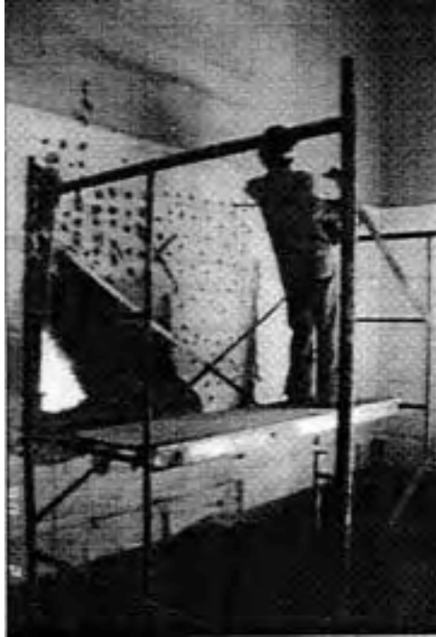
Drilling reinforced concrete wall before removal from adjacent historic fabric in Ballajá Military Barracks in Old San Juan, PR (1988).
