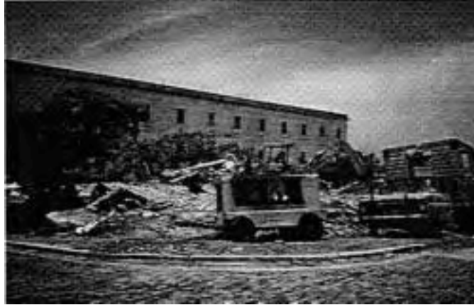
Demolition of existing structures for Plaza Quinto Centenario in Ballajá District of Old San Juan, PR (1986).
