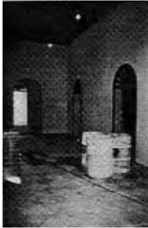
Restoration of interiors of Casa Ramón Power y Giralt as headquarters of the Conservation Trust of Puerto Rico (1995).
