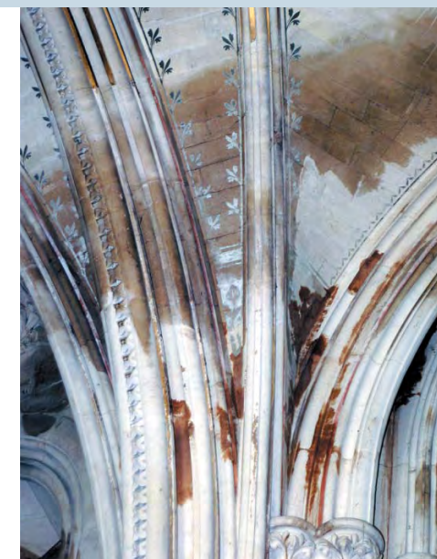
Tyntesfield is another property where there has been water penetration. [SPAB/Peter Robins]
