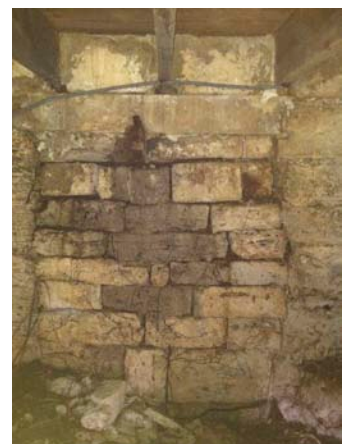
below: Blocked door from patio to the cottage cellar
