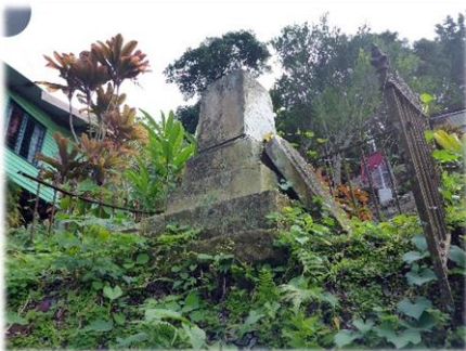
The erosion is clearly visible
