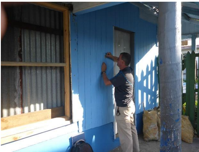
Front of the building with sampling site on the vertical wall lining.
