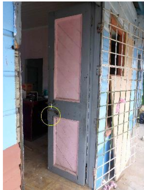
Right door with location of broken lock stile
