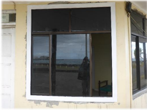
Example new aluminum window frame
