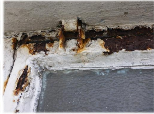
Original corroded steel window frames.
